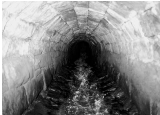
Figure 8. Stone-built culverted watercourse between the New Pool and the Upper Furnace Pool, one of the earliest elements of the culvert system dating to the 18th century (Photograph by OnSite Surveys, reproduced courtesy of the Borough of Telford and Wrekin).
