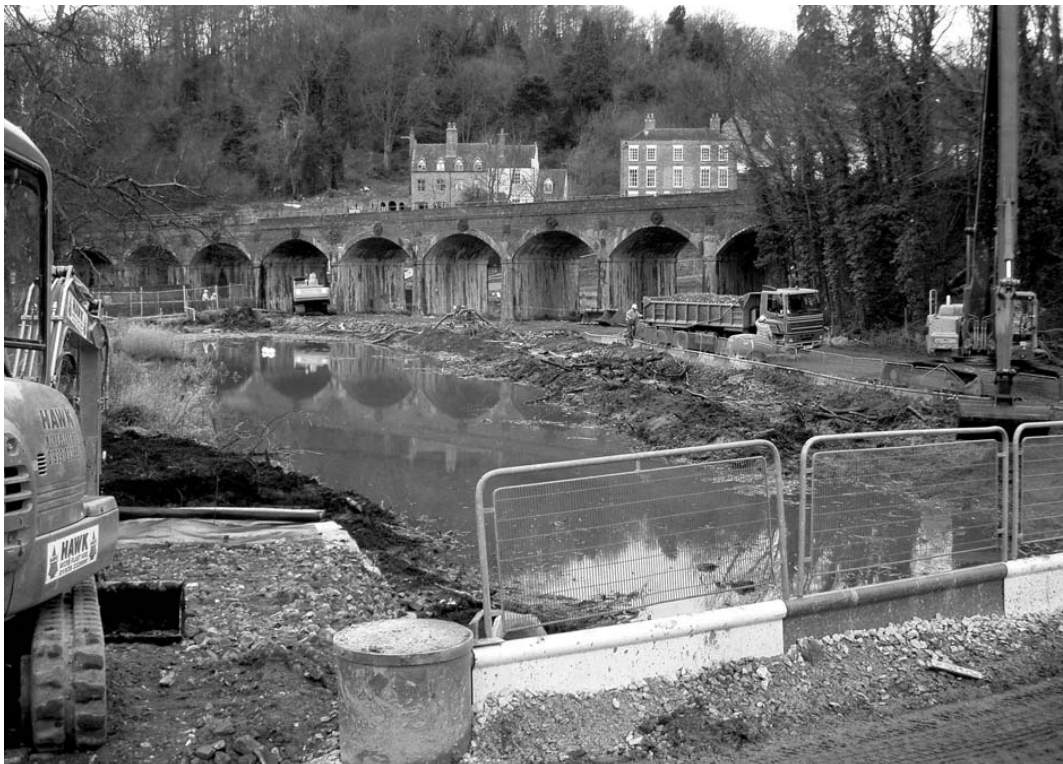
Figure 15. Upper Furnace Pool during the first phase of desilting operations in 2004. The haul road has been constructed into the centre of the pool (in front of the viaduct) to enable plant to access the southern part of the pool (Photograph by Paul Belford).
