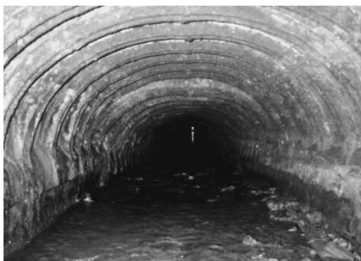
Figure 11. Iron-framed brick culvert section of the former Upper Forge Pool, which was culverted piecemeal during the expansion of the works in the 19th century (Photograph by OnSite Surveys, reproduced courtesy of the Borough of Telford and Wrekin).
