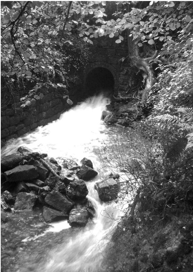
Figure 20. The outflow of the culvert between the New Pool and the Upper Furnace Pool, probably constructed in the late 18th century (Photograph by Paul Belford).
