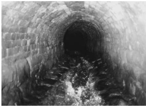
Figure 9. Stone-built open watercourse later culverted in brick, between the New Pool and the Upper Furnace Pool (Photograph by OnSite Surveys, reproduced courtesy of the Borough of Telford and Wrekin).
