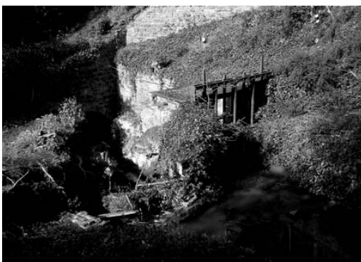
Figure 12. Upper Forge Sluices in 2005, prior to restoration. The main sluices were blocked by landslip and other debris, and the water had forced its way past the structure, collapsing an early overflow culvert to the east (Photograph by Paul Belford).
