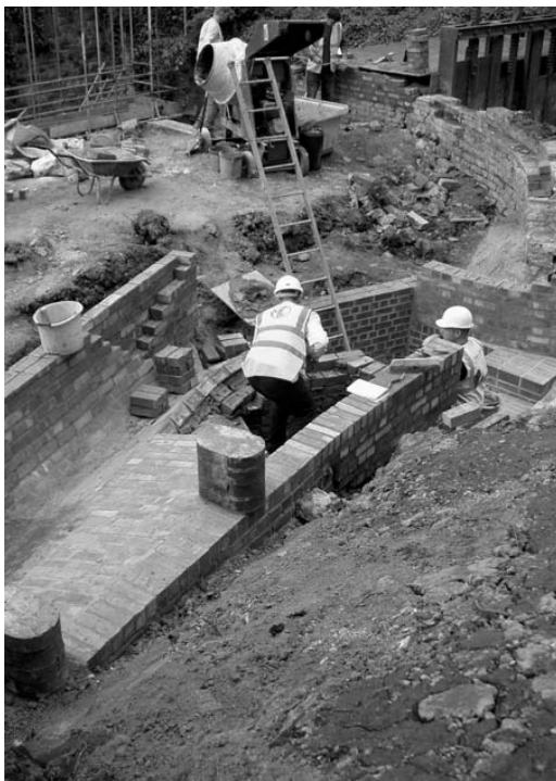
Figure 13. Upper Forge Sluices during restoration work in 2006. The original overflow structure is being rebuilt to the original design, and the culvert into which it originally fed, which had collapsed after many years of neglect, was reinstated to modern specifications (Photograph by Paul Belford).
